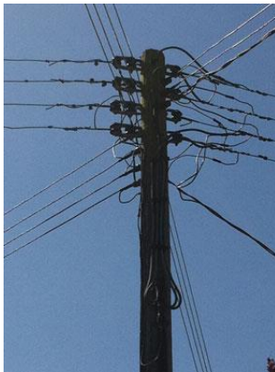
Open bare conductors
